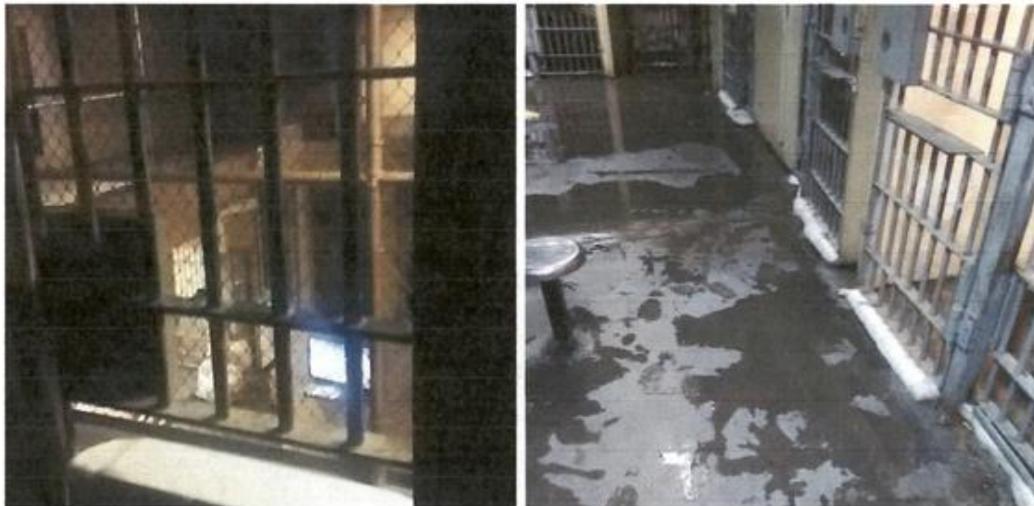
Mississippi State Penitentiary at Parchman. Left, hundreds of Parchman inmates sit in the dark because their lights don't work. Right, Parchman inmates say toilets sometimes back up and overflow during the rain.
